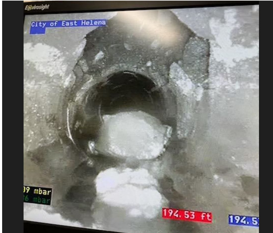
Top of Pipe Missing in American Chemet Service Crossing
