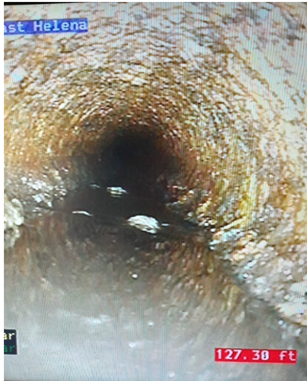
Corrosion and Debris in Manlove Sewer Crossing
